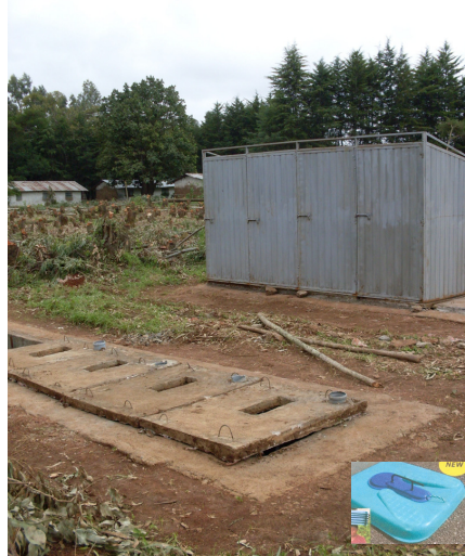
First 4 toilet stalls in place. Next 4 toilet floors await plastic squat toilets and metal stall structure.
